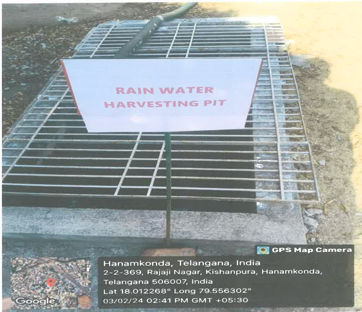
Rain Water Harvesting Pit:
