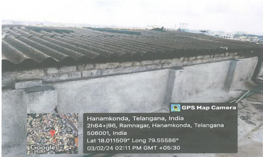
Tanks and Bunds
