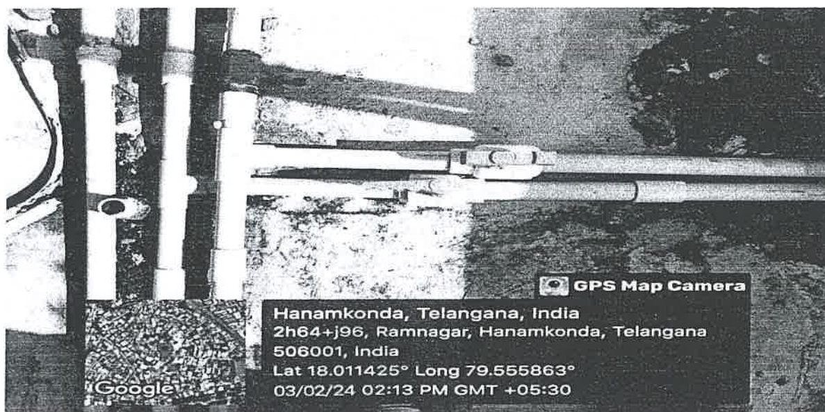
Water Distribution Systems in the College from the Tanks
