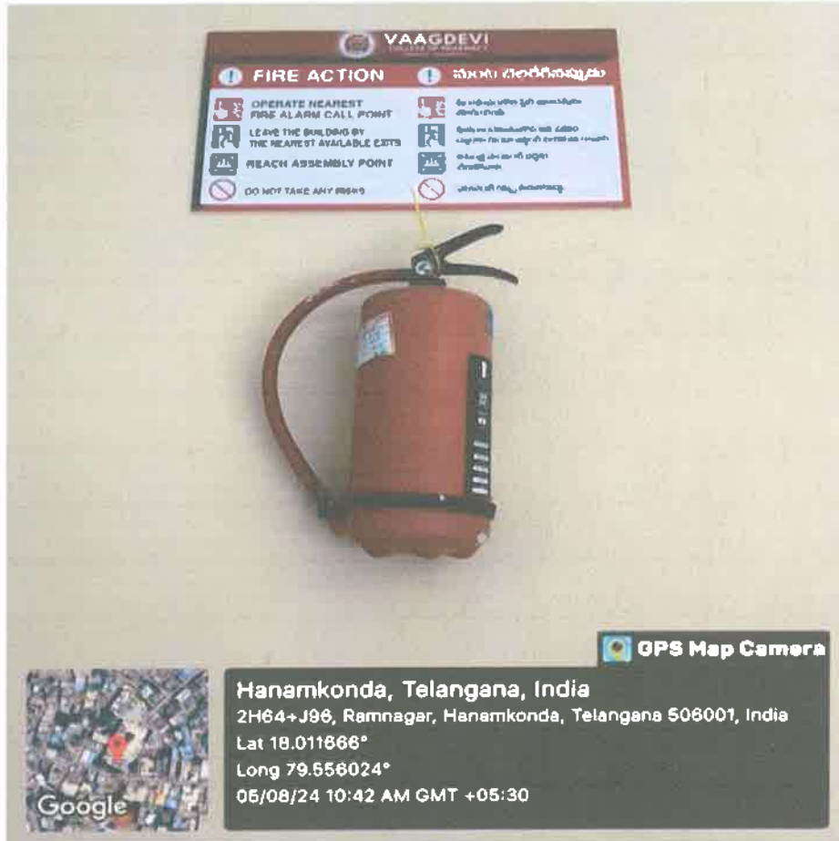
Plate 1: Fire extinguishers in the premises
