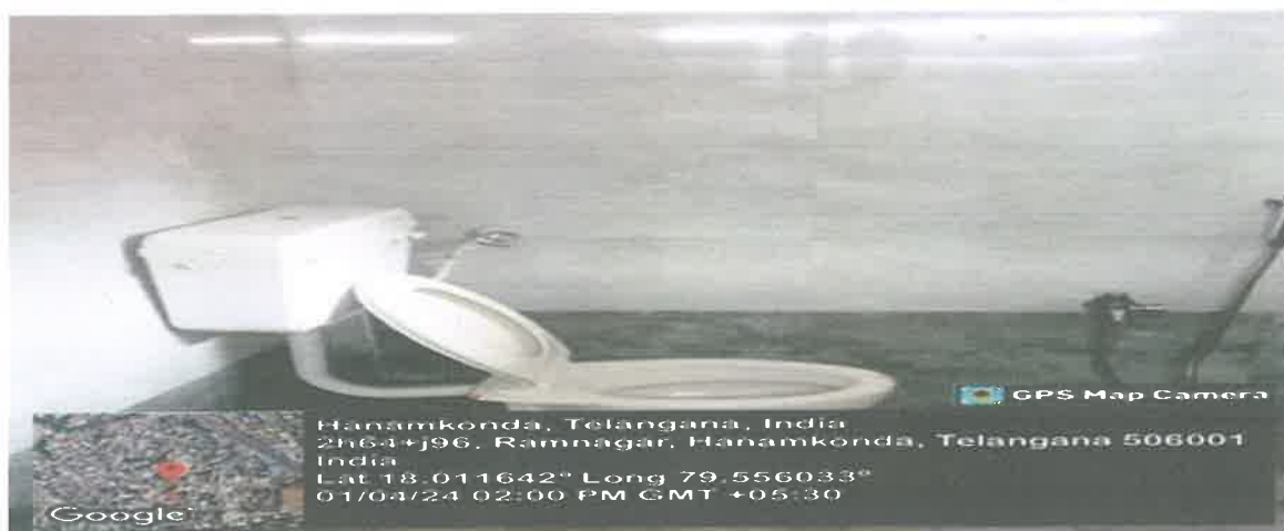
Divyangjan Friendly Washroom
